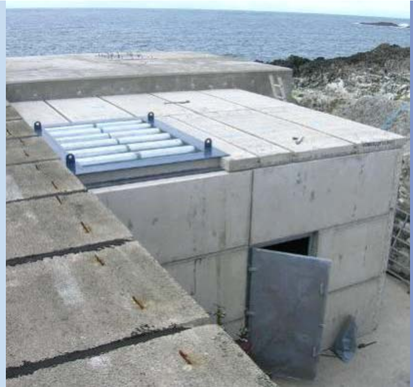
Turbine hall & acoustic attenuator
